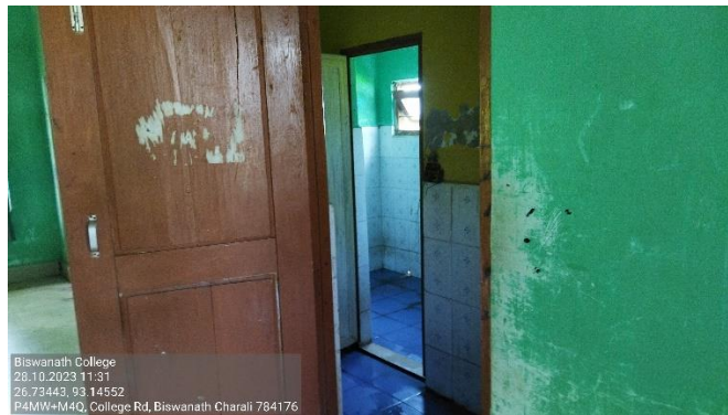
Girl's Common room equipped with Sanitary Napkin Vending Machine and toilets
